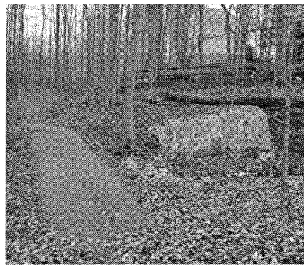
Improvements to the community's paths included this upgrade to the culvert area near the tot lot.
